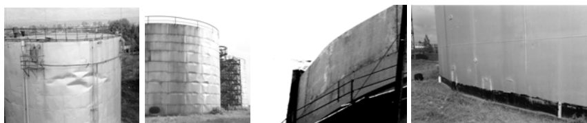
Fig 1. Examples of local shape defects of steel cylindrical tanks
