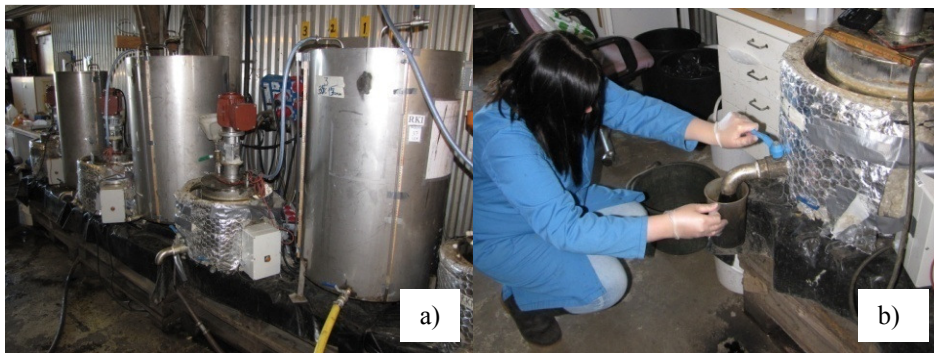
Fig. 2.4. a) Pilot-scale digesters located at Sjölanda wastewater treatment plants (Malmö, Sweden); b) manual operation of reactors.
