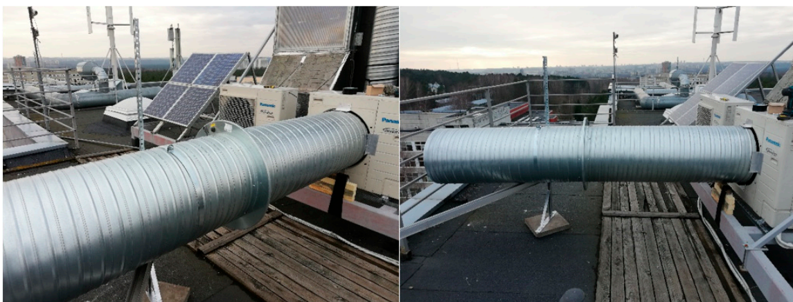
Figure 2. The experimental setup on the roof of VILNIUS TECH.
