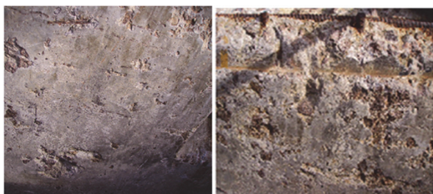
Fig. 1. Damages in concrete surface of a hydraulic structure.
