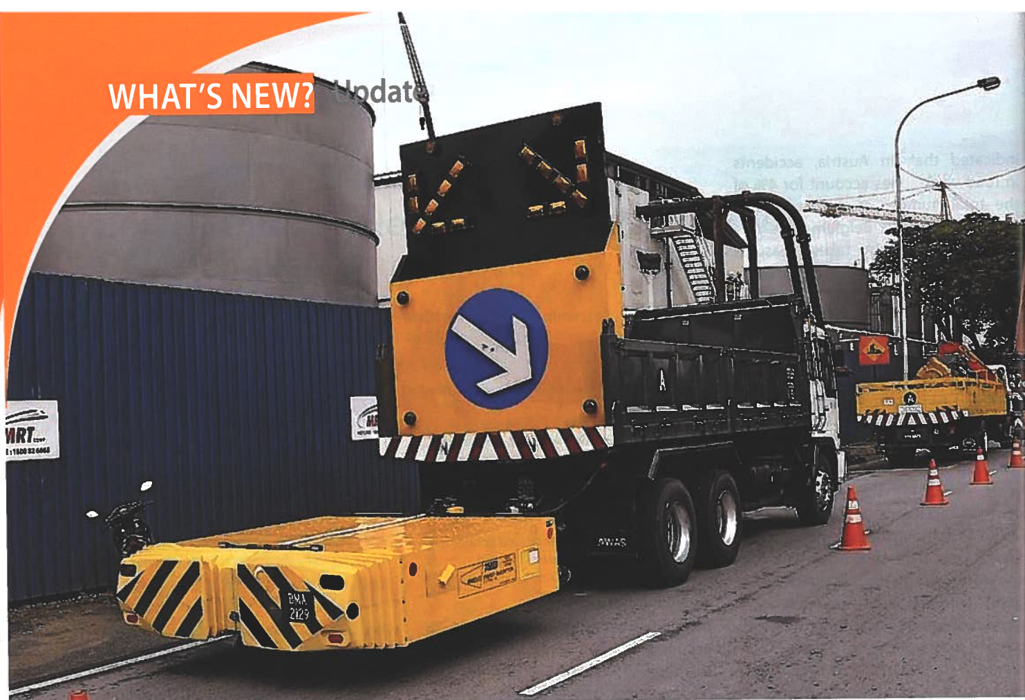
Illustration 5 - Safety measure in road work zone: lorry-mounted attenuator © www.thestar.com
