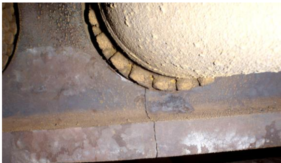
Fig. 2 Tube coil sheet fractures
