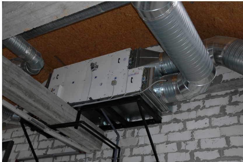
Fig. 2. AHU with AC motors
