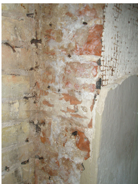
Figure 3. Efflorescence of salts on inner wall
