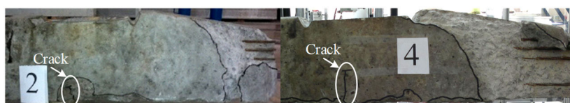
Figure 3. Damaged ends of exploited sleepers
