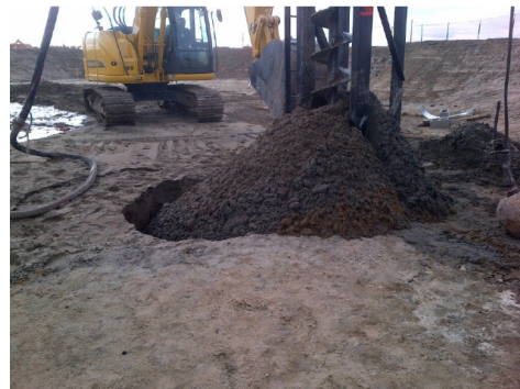
Fig. 2. Drilled soil mass by the auger and settlement trough in the vicinity of the boring location
